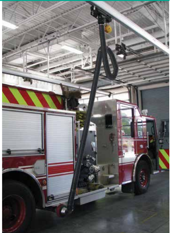
Hollywood, Florida, F.D. now uses Masterduct Fire Flex® dual temperature hose to exhaust high-temp fumes from newer engines. Upper hose section, above safety disconnect, is a multi-ply hose for maximum flexibility, strength, and temperature resistance
